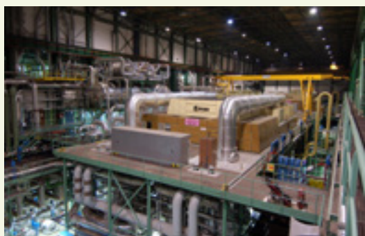
2011: Turbine hall with turbines © Javys.
