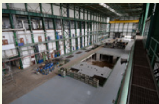
2015: Turbine hall without turbines © Javys.
